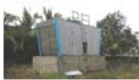
TIMBER COOLING TOWERS
