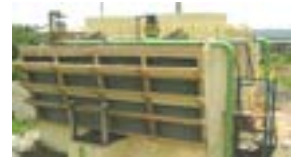
RCC COOLING TOWER
